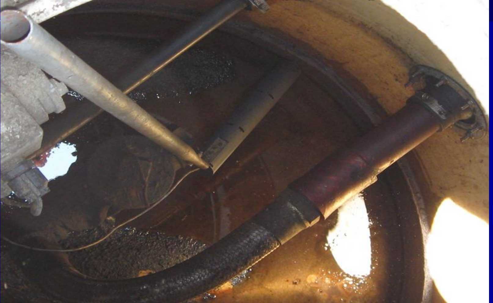
Sensor is mounted wrong and wrong position
