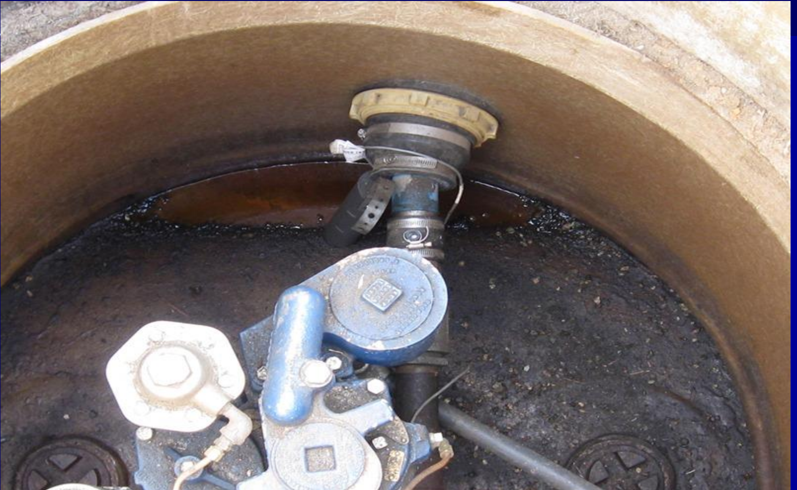
Sensor in wrong location and not picking up leak
