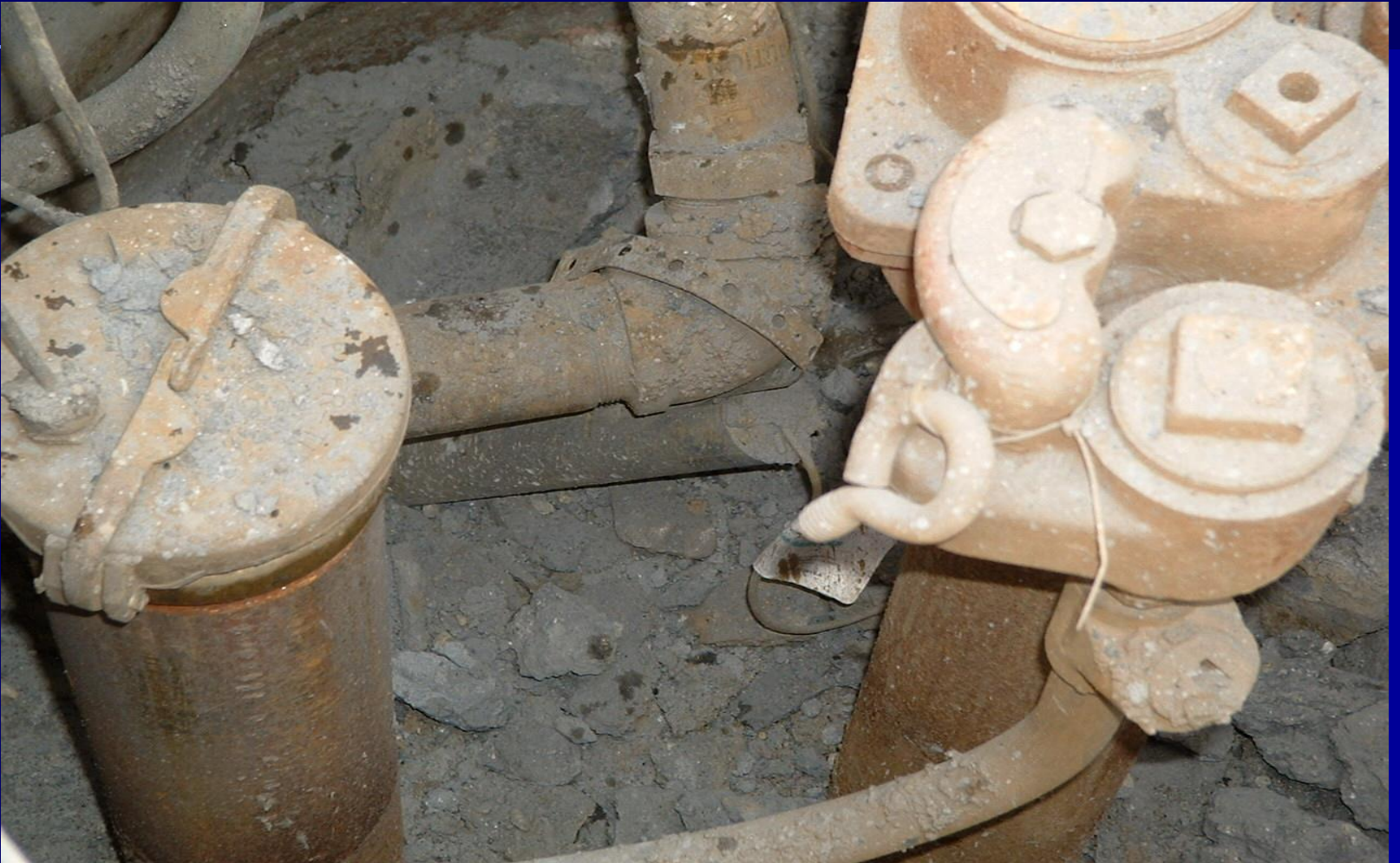
Sensor in wrong location and not properly mounted
