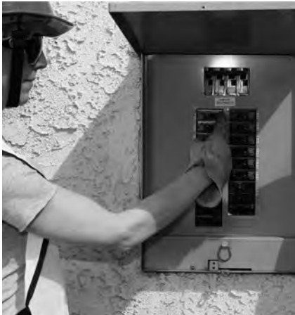
Step 1: Turn off individual breakers one at a time
